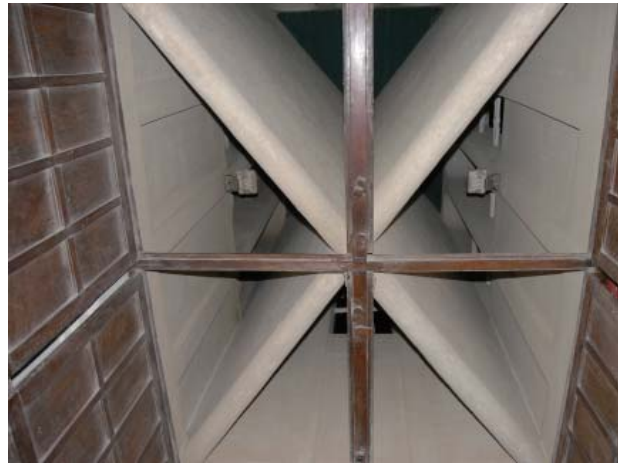
Fig.92 Inner structure of the wind tower of Shaikh Isa Bin Ali House
