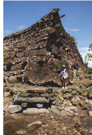
Photo 18 Crack in the massive basalt boulder in the southeast corner of the outer wall
