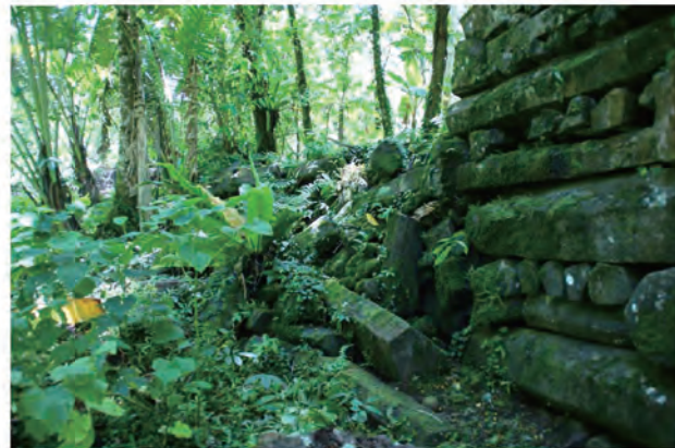
Photo 3 Collapse of the northeast outer wall
