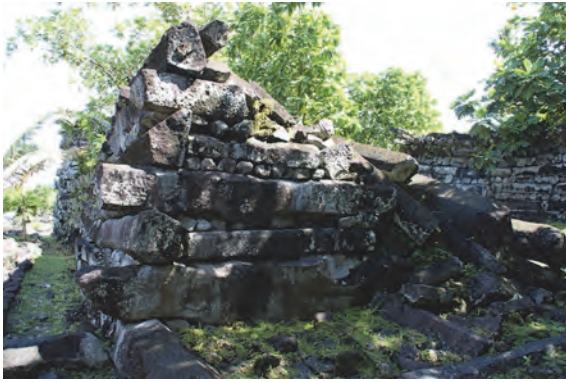
Photo 15 Collapse of the perimeter wall on the north side of the entrance
