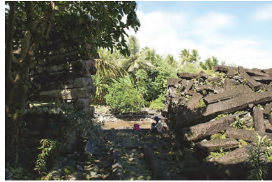
Photo 16 Collapse of the entrance and perimeter wall seen from the inside
