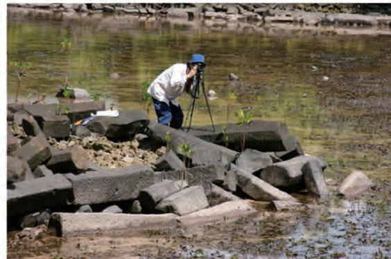
Photo 7 Collapse of the northeast corner of the stonewall on Dau
