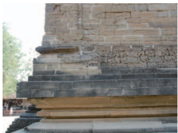
Fig.28 Original sandstone materials that have deteriorated (top portion) and newly replaced materials (bottom portion) at Nan-hpaya
