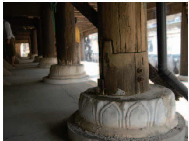
Fig.61 New plinths and pillar bases that have been repaired at Shwei-nan-daw Monastery
