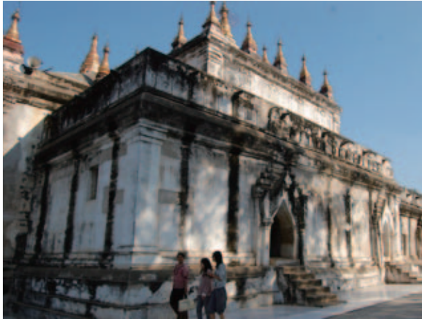
Fig.29 External view of Ma-nu-ha-hpaya and traces of where reinforcement materials have been inserted in the wall corner
