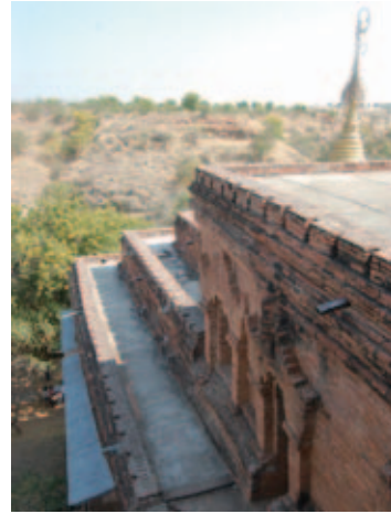
Fig.13 Drainage facility seen from above Kyauk-ku-umin
