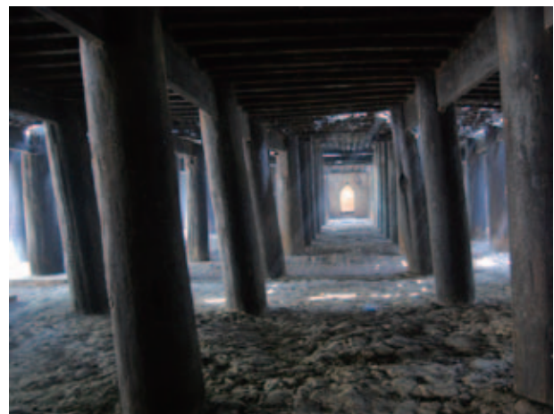
Fig.79 Tilted pillars and sedimentary sand and soil beneath the floor at Bagaya Monastery
