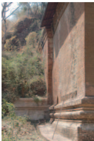
Fig.16 Bulging of the outer wall of the east façade of Kyauk-ku-umin
