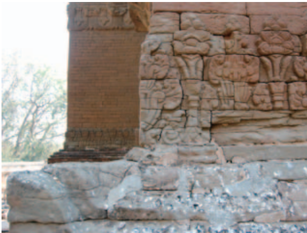
Fig.14 Deterioration of the lower sandstone portion of the outer wall of Kyauk-ku-umin
