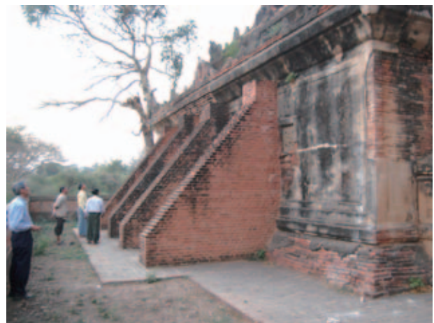
Fig.40 Buttress reinforcements on the outer wall of the south façade of Pitakat-taik
