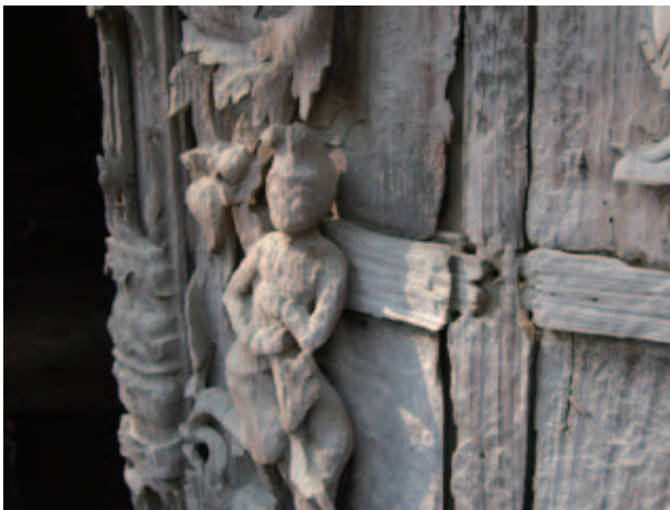
Fig.58 State of deterioration of the walls of Shwei-nan-daw Monastery
