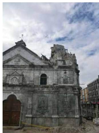
Fig.87 Collapsed belfry of Basilica Minore del Santo Niño after earthquake
