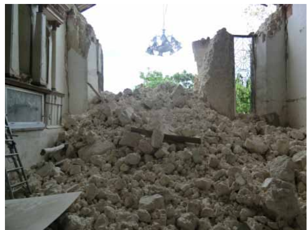
Fig.123 Collapse of Santo Niño Church after earthquake
