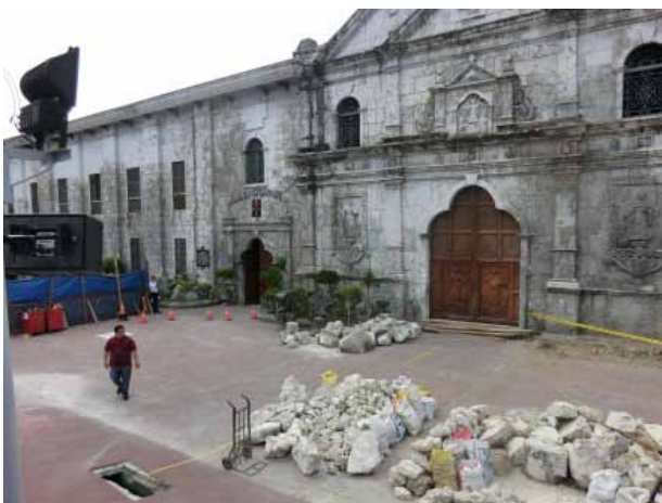
Fig.86 External view of Basilica Minore del Santo Niño after earthquake
