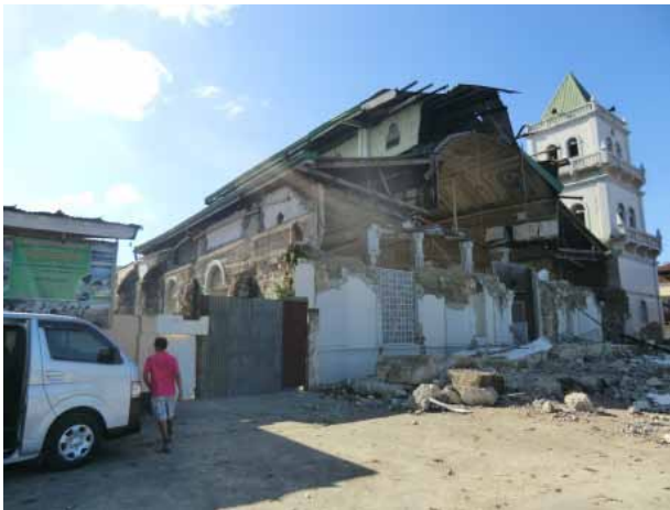
Fig.114 Church of Isidore the Farmer after earthquake
