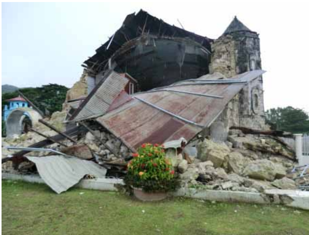
Fig.126 External view of Church of San Pedro after earthquake
