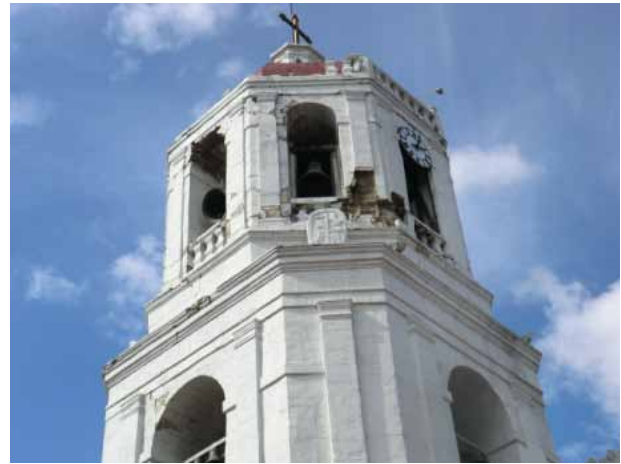
Fig.89 Crack in belfry of Cebu Metropolitan Cathedral after earthquake
