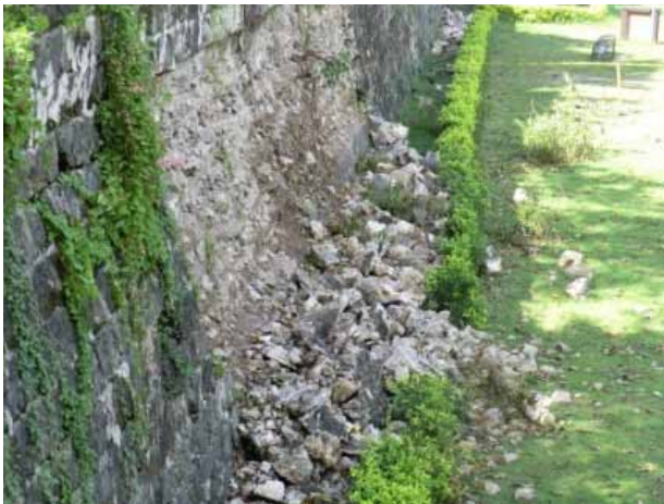
Fig.84 Destroyed stone wall of Fort San Pedro after earthquake
