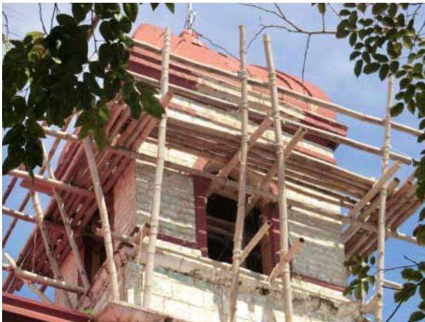
Fig.96 Restoration of crack in the belfry of Church of Santa Catalina de Alejandria after earthquake
