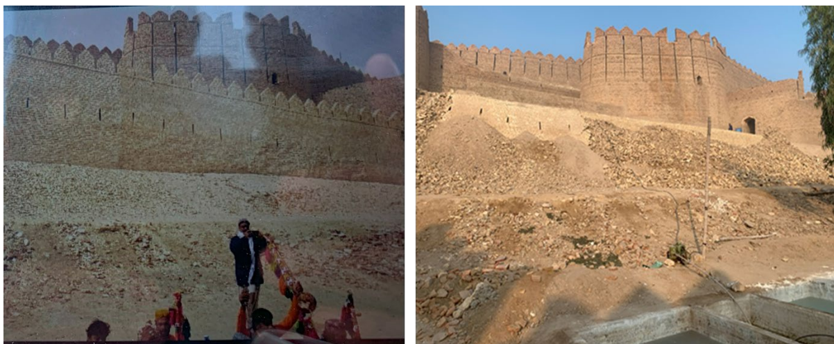
Fig. 3 Left image depicts the previous condition of the boundary wall (source: Bilawal) right image depicts the status of the boundary wall near of the entrance
