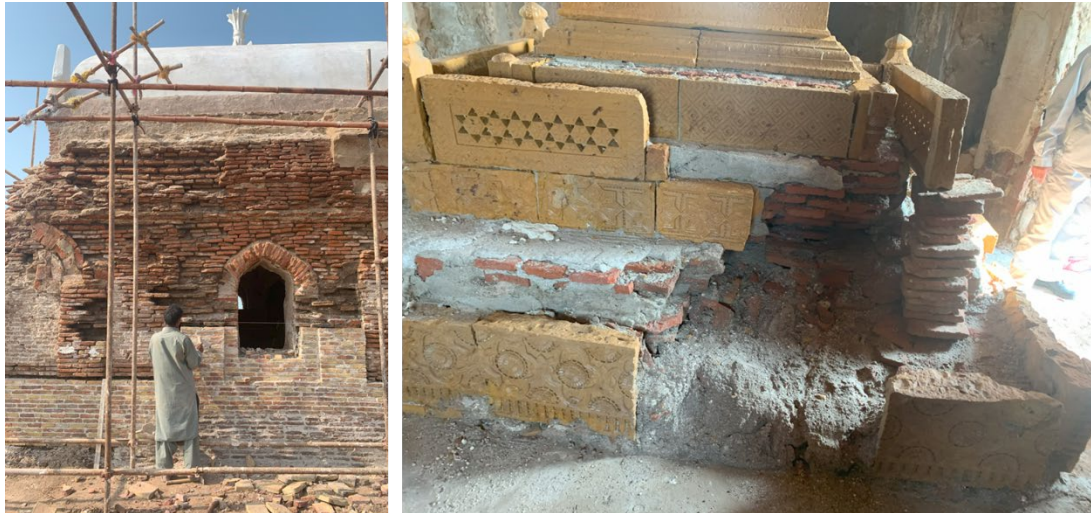
Fig. 3 Outer renovation and restoration works and damages to the grave structures due to dampness
