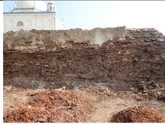
Fig.8 On the north face of the north wall (opposite side of Fig. 7), salt weathering is observed.
