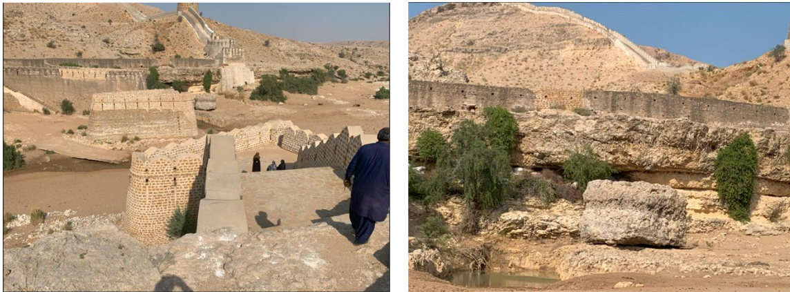
Fig. 3 Flow path of Sann river near the main gate and the eroded condition of the wall foundation and supported by sand bags
