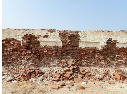
Fig.7 Partial brickwork collapse is observed on the south face of the north wall.
