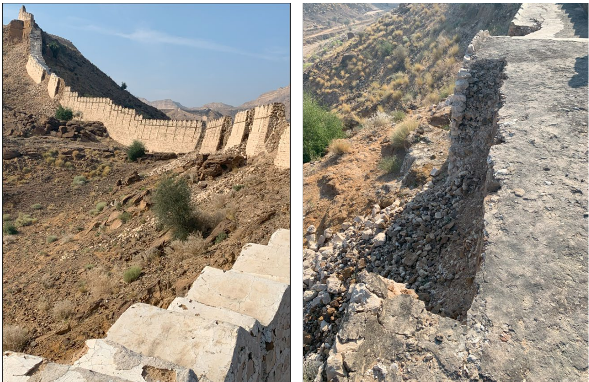
Fig. 1 Damages to walls and basements
