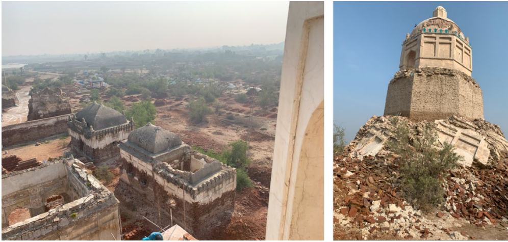
Fig. 4 Damage status of the domed structures/tombs
