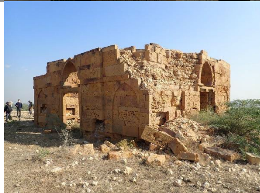
Fig.3 The building is mainly constructed of stonework; strong rainfall during the flood of 2022 caused the building to collapse.
