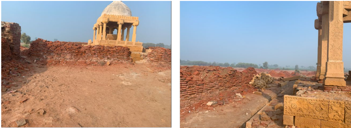
Fig. 2 Status of the walls and structures after the damage
