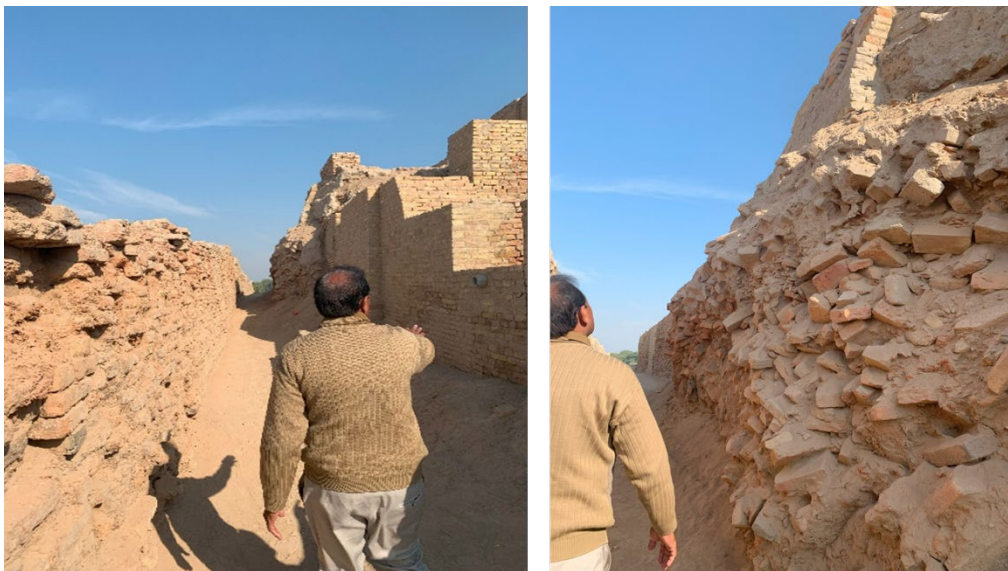
Fig. 3 Left image depicts the status of the ruins and conservation of wall basements using mud and straw and right image depicts the collapse of the structure and wall which need to be restored later with proper care.
