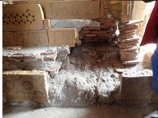
Fig.6 Fig. 5 Lower part of the tomb enshrined in the mausoleum on the left. Salt weathering is significant.
