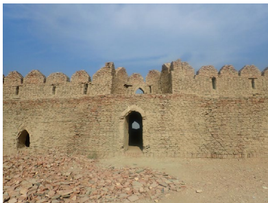
(a) West side (Major damage)
