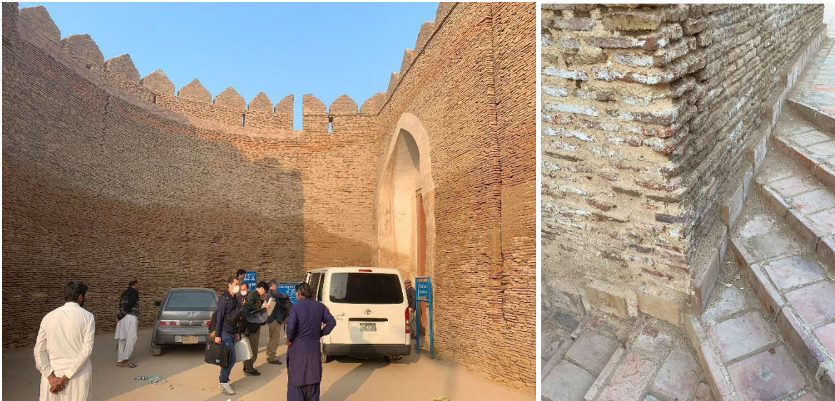
Fig. 2 Left image depicts the entrance to fort and right image depicts the status of the boundary wall near of the entrance
