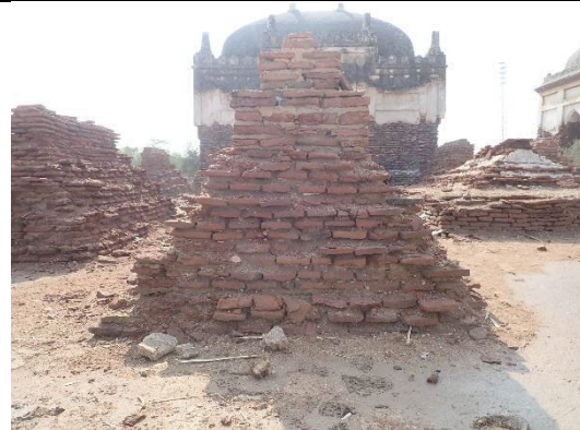
Fig.9 Brick tomb. The condition of the north face is not as severely deteriorated as the east, south, and west faces.
