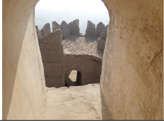
Fig.6 The plaster layer in the roof area at the back of the figure is fragmented and has lost its waterproofing function.
