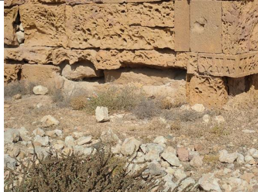
Fig.6 Salt weathering observed in the lower part of stonework structures.
