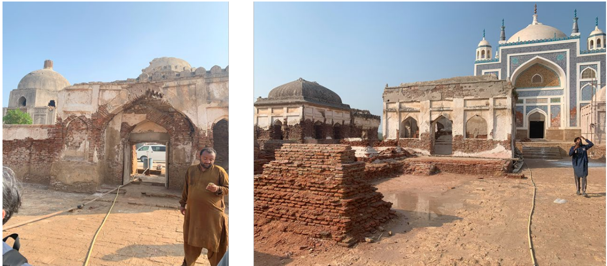
Fig. 2 Status of the walls and structures after the damage
