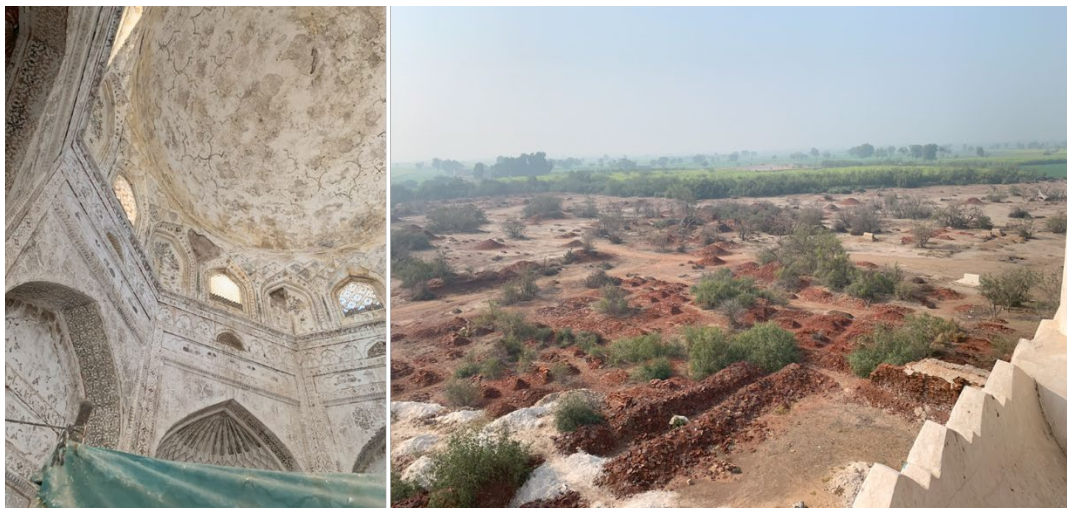
Fig. 3 Cracking on the main dome and damages to the surrounding graves
